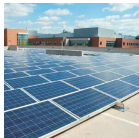
A look at AstraZeneca's 7,300 solar panels that were installed in June at its Wilmington, Del. campus
