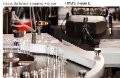
isolator, the isolator is supplied with conditioned air for Zone A via unidirectional air flow. The return air from the isolator to the recirculation fan travels through the double wall of the isolator (1). Spread of released HPAPIs from the isolator to the isolator plenum is possible, thus the classic isolator is not suitable for the use of HPAPIs (Figure 1).
